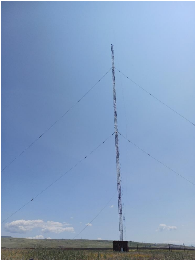
Photo 8 – The primary support structure used at EK8A for the newly installed wire antennas.
