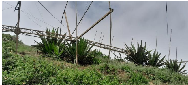
Collapsed 15-meter tower at D4C that was quickly repaired for the contest.
